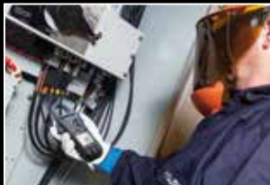
Analyze power-related issues
