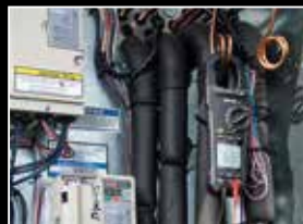
Diagnose VFD-controlled problems
